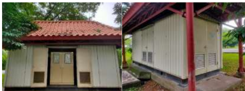
Gambar 1.1 Gardu RB Bandara Internasional Juanda
